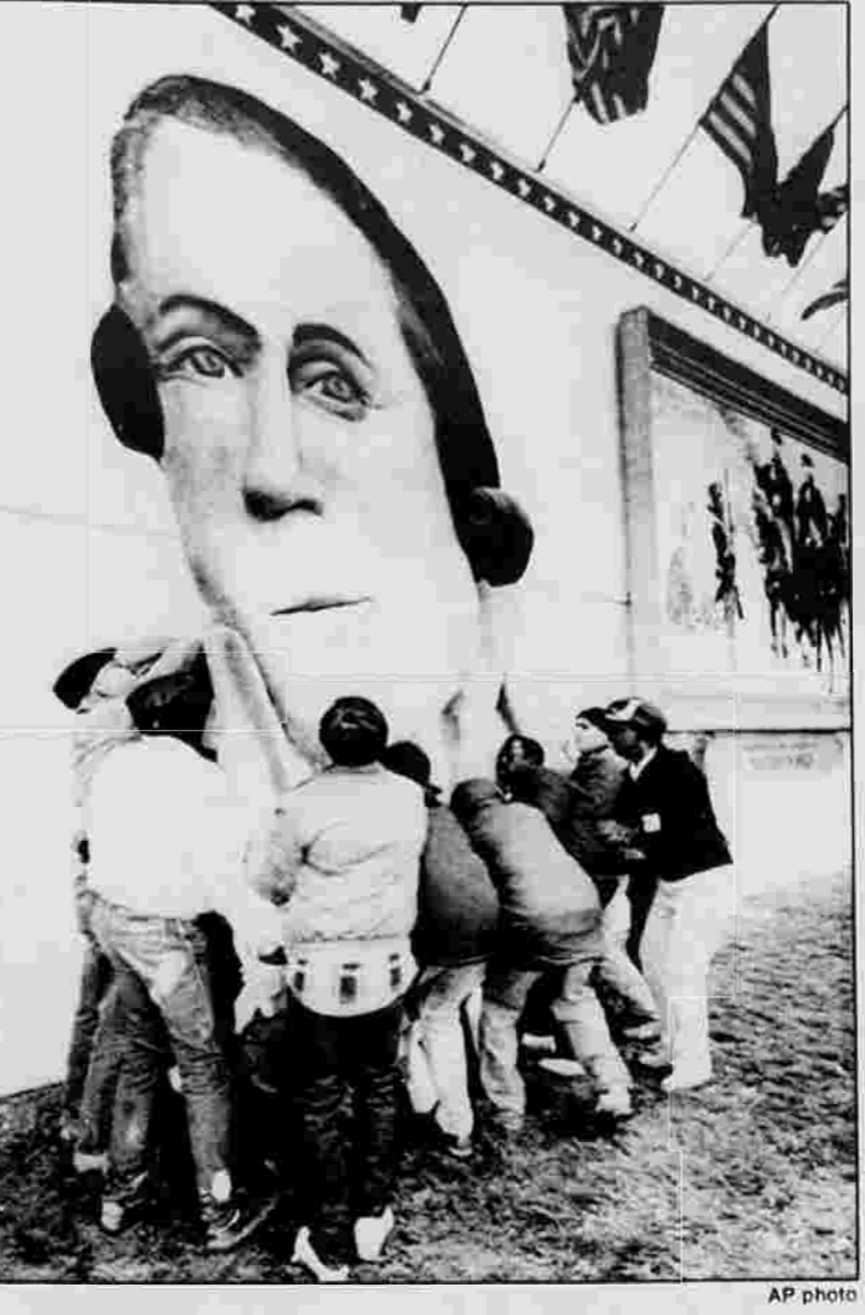
INAUGURAL PREP — Workers stand up a 16-foot bas-relief of George Washington on the Mall in Washington in preparation for Friday's inauguration of George Bush. One of the 9-by-12-foot paintings of key events in U.S. history is at right.
